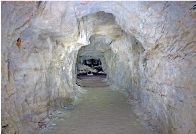
Unlined tunnel in Objekt C showing the weakness of the bedrock. A rockfall is visible in the distance
